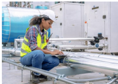
Cool room pipe work
